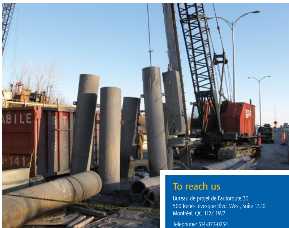
Work on the temporary railway overpass on the A-15 in Candiac is now most visible.
