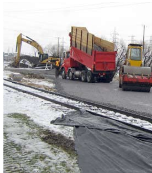
Installation of membranes and crushed stone in preparation for the construction of the railway.
